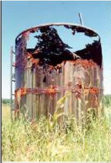
A brine tank in Chautauqua County in need of repair
